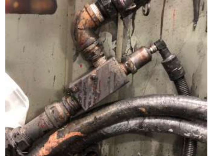
Showing the installation of an inline viscometer in an ink delivery system
